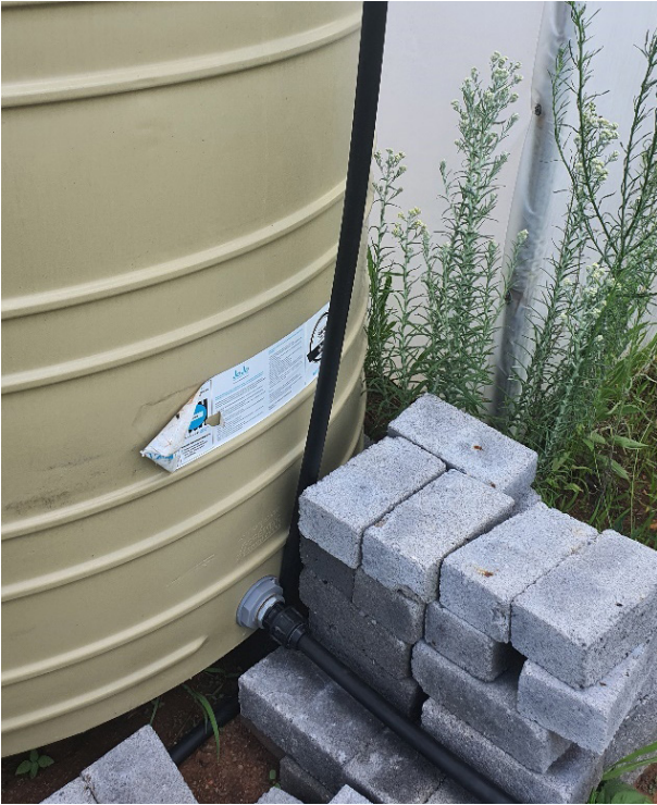
1. Water supply system funded by UN Women Climate Smart Agriculture (CSA) Project, Tumahole, Parys, Free State
