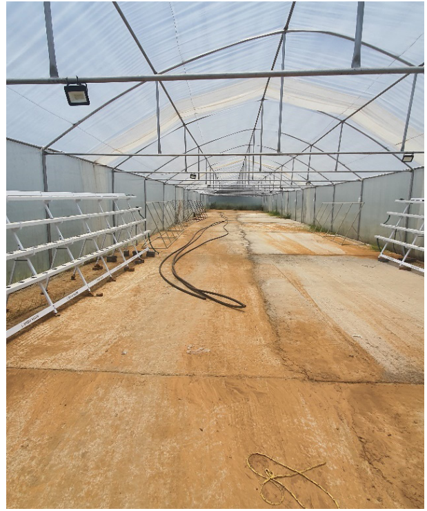
2. Inside the incomplete tunnel erected for the project, Tumahole, Parys, Free State
